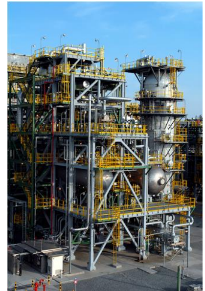
Example onshore amine plant
